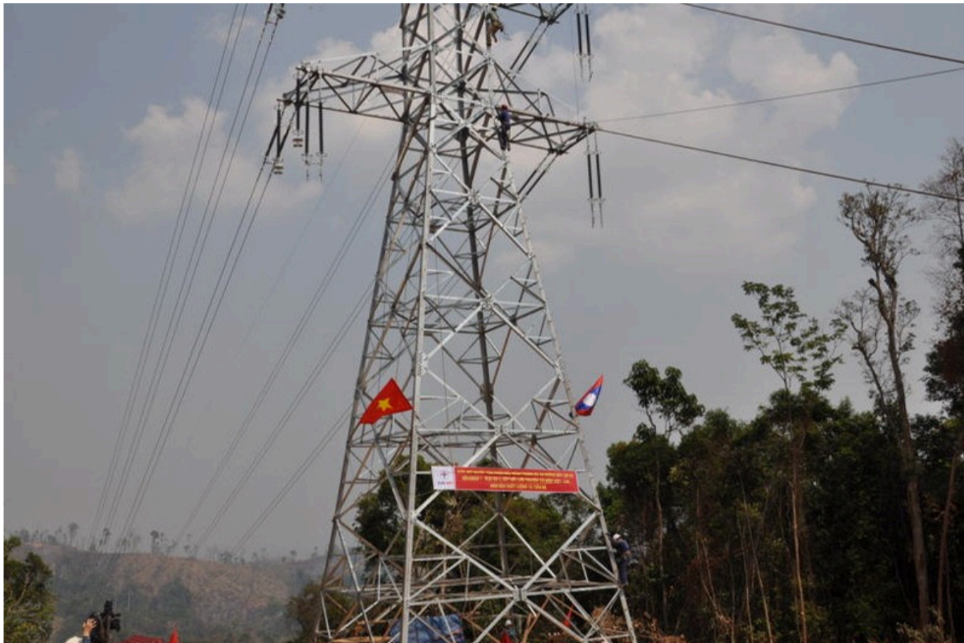
A part of the 220 kV power line connecting Laos and Vietnam in Gia Lai province, Vietnam's Central Highlands. Photo courtesy of EVN.
